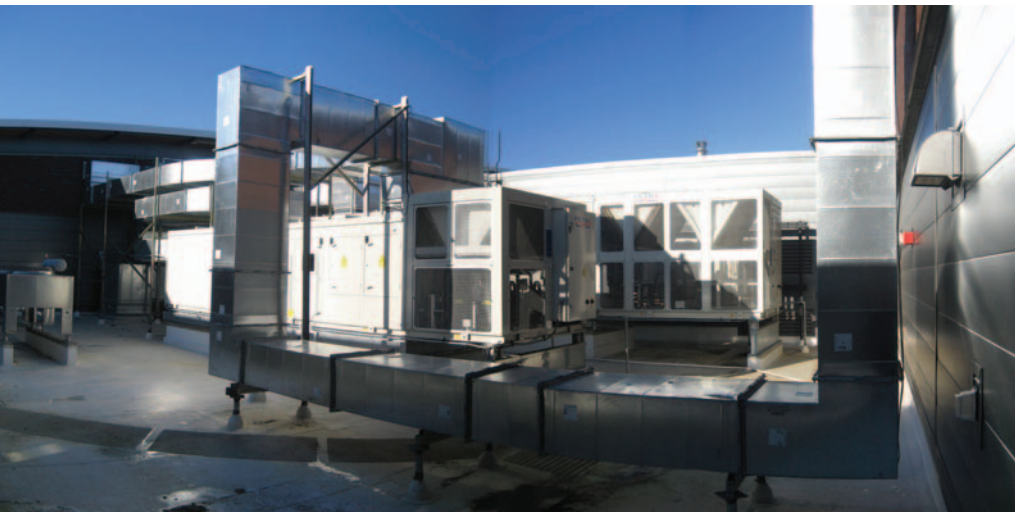
A view of UVC-equipped air handlers at Sammamish Commons in Washington, the first HVACR project to earn a LEED point for the use of UVC lights.
