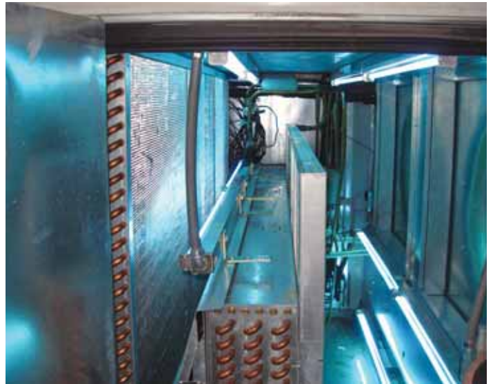
Eco-Care, a company specializing in pollution control and energy conservation, installed UVC lights, on a phased basis, in three air-handling units serving the ASPCA building in New York City.
