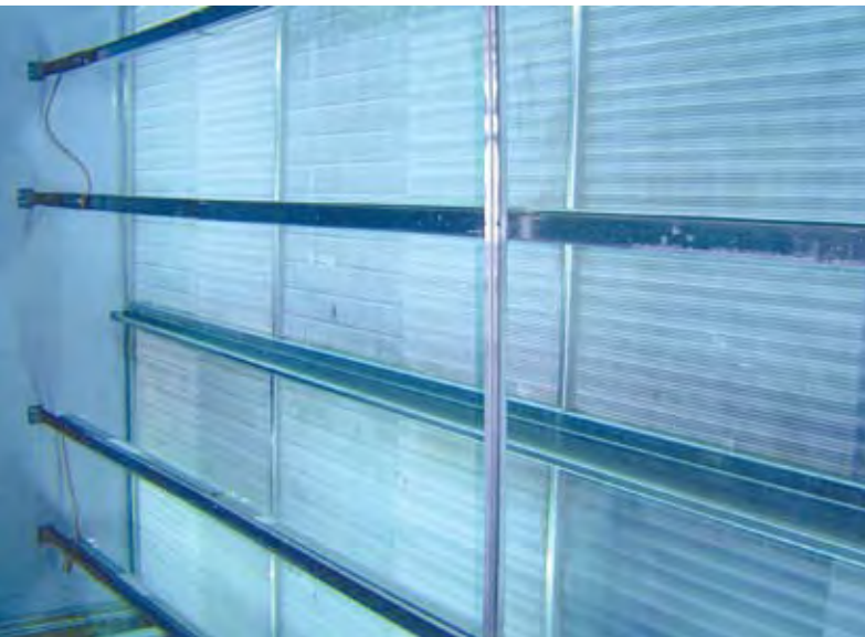
UVC Emitters™ shining on a hospital A/C coil.
