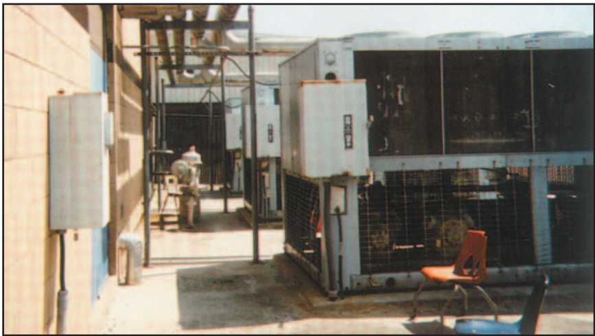
The chiller plant on the Rizzuto Elementary School campus.
