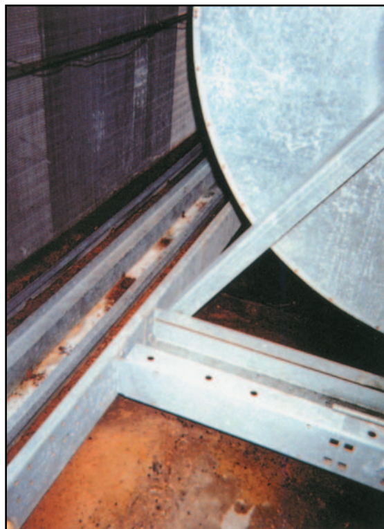
A close-up view of the air handler at Jennie Reid Elementary School.
