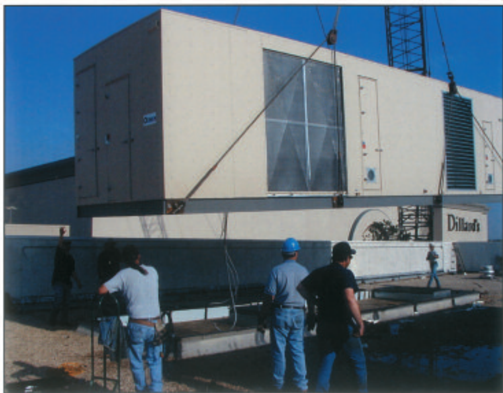
The retrofit was challenging because the mall was on a very tight schedule and at the time of the retrofit, an evening thunderstorm could pop up at any time.
