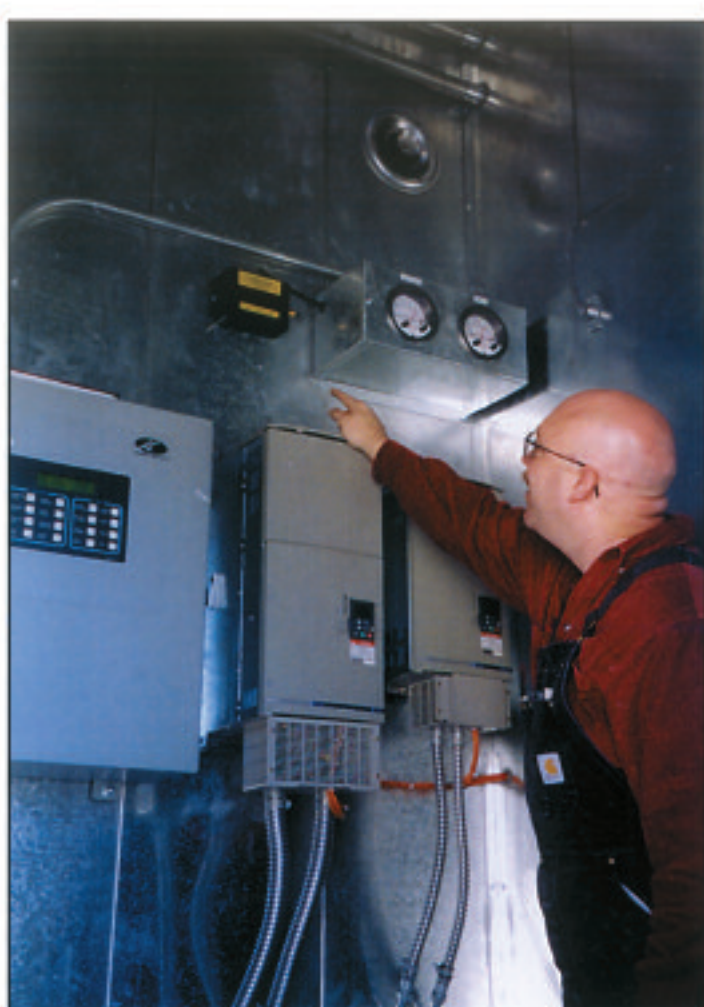
A mall maintenance person examines the radiometer used to measure UVC output and ensure that the devices are working properly.
