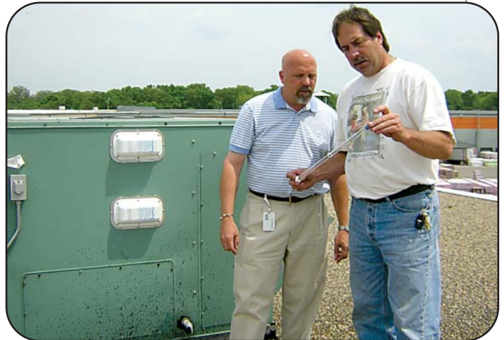
Bruce Strandberg (left) and Randy Remer prepare for annual changeout of the replaceable UVC Emitter™ tubes in the rooftop air handling units.
