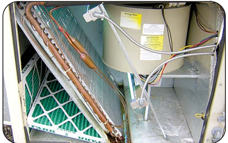
UVC Emitters™ in the air handling units have successfully eliminated both surface mold and airborne mold spores at Medicine Lake Properties.
